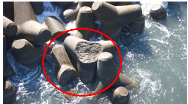
Fig.11 Broken blocks which are relatively new
