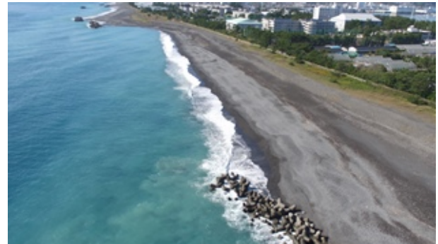
Fig.9 Erosion proceeds between block areas
